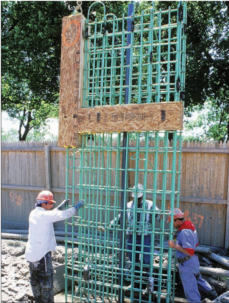
Workers lower the reinforcing cage for the slurry wall. The green color of the bars indicate their epoxy coating.
